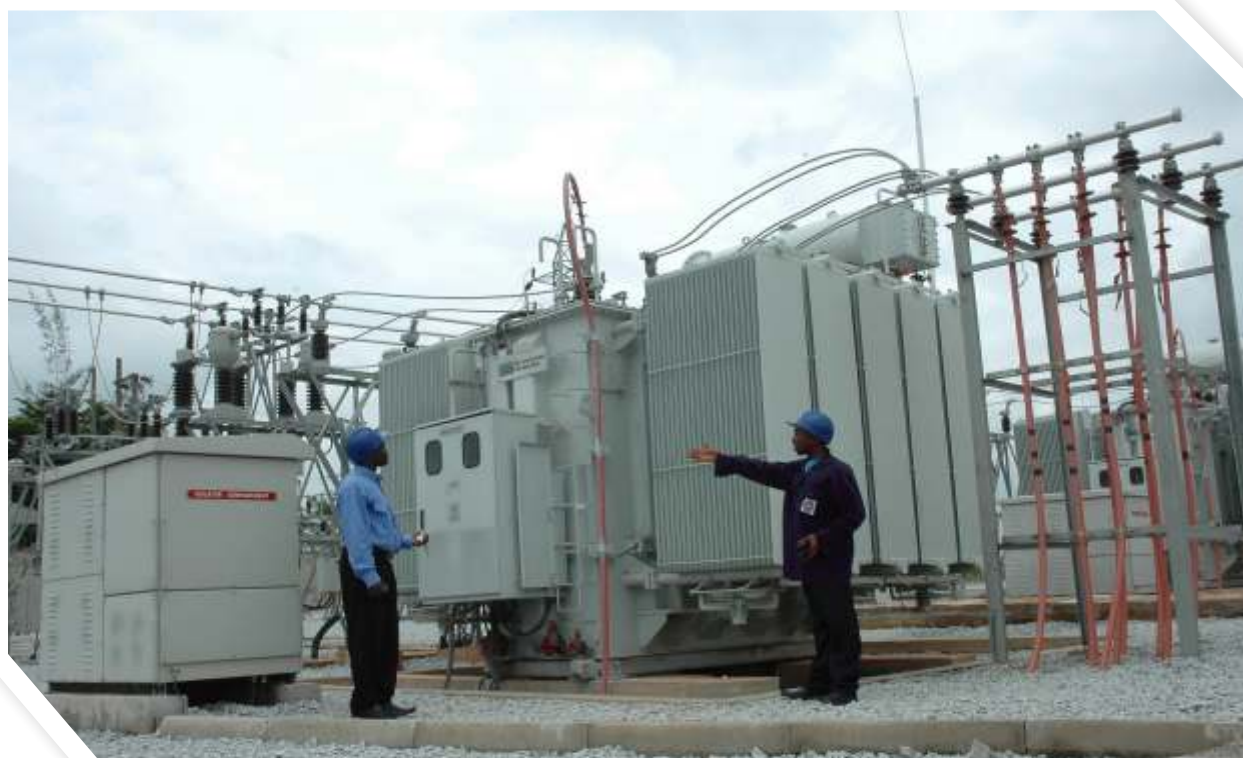
A New Transformer to Meet Growing Demand
